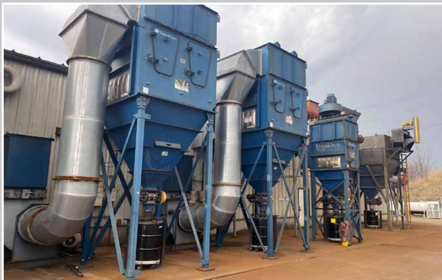
View of Dust Collection System
