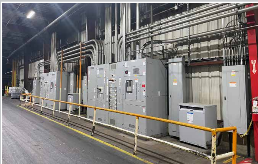
View of Electrical
